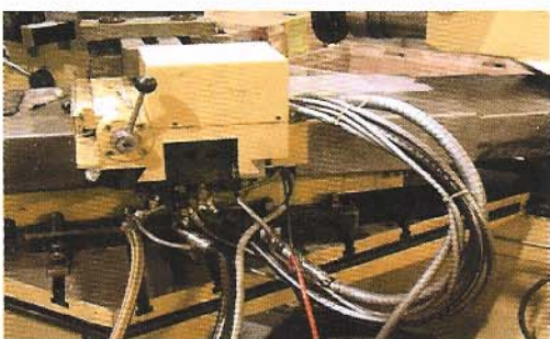
Electrical Cable Armour
